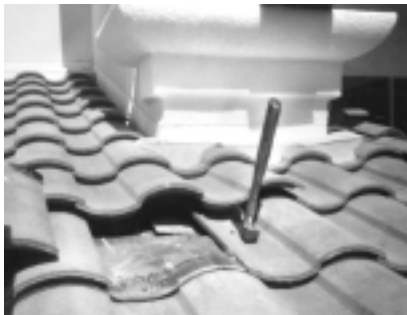
Defects revealed thru investigative tests
