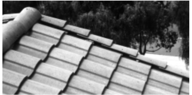
Poorly installed rake tiles and debris indicate potential problems
